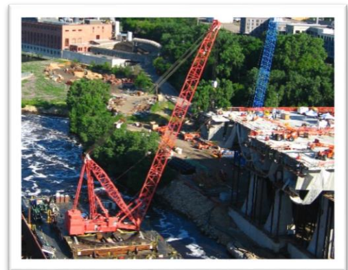
Ringer cranes were used to build the new I-35W bridge in Minneapolis, Minnesota.
