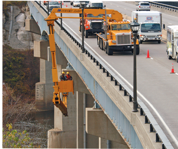
Under-bridge inspection vehicles pose safety risks to workers and are expensive to purchase and operate.
