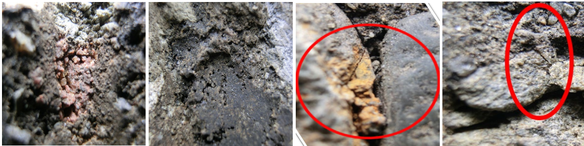
Figure 4.6 Crushed, missing, and cracked materials in HMA from layer below milling depth.
