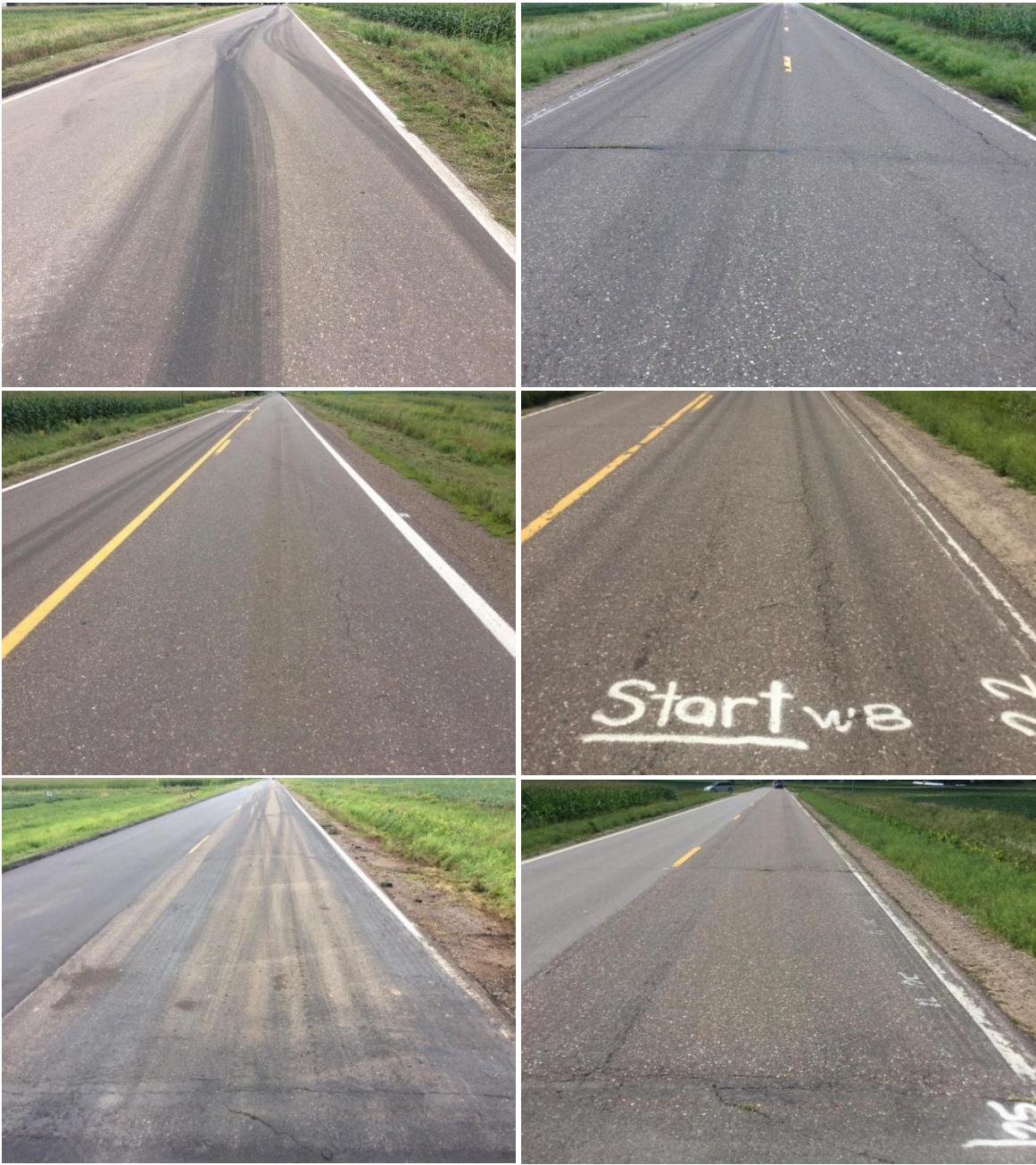
Controls: Cell 8021 (top), 8022 (middle), 8025 (bottom) inspected in 2016 (left) and 2020-21 (right).
