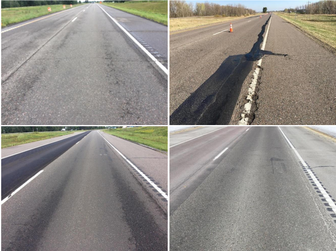
Controls: Cell 169000 (top), 169014 (bottom) inspected in 2016 (left) and 2020-21 (right).
