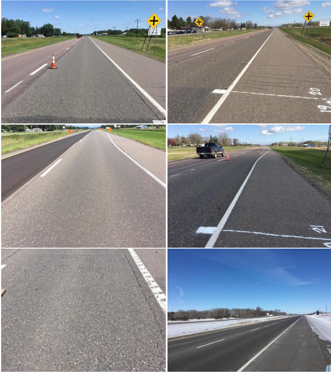
Controls: Cell 169020 (top), 169021 (middle), 169028 (bottom) inspected in 2016 (left) and 2020-21 (right).
