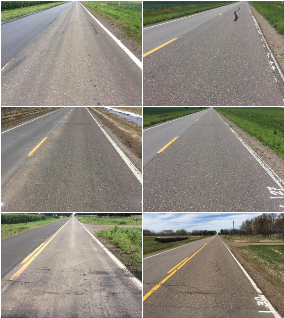
Controls: Cell 8026 (top), 8027 (middle), 8030 (bottom) inspected in 2016 (left) and 2020-21 (right).
