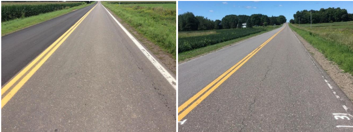
Controls: Cell 8031 inspected in 2016 (left) and 2020-21 (right).
