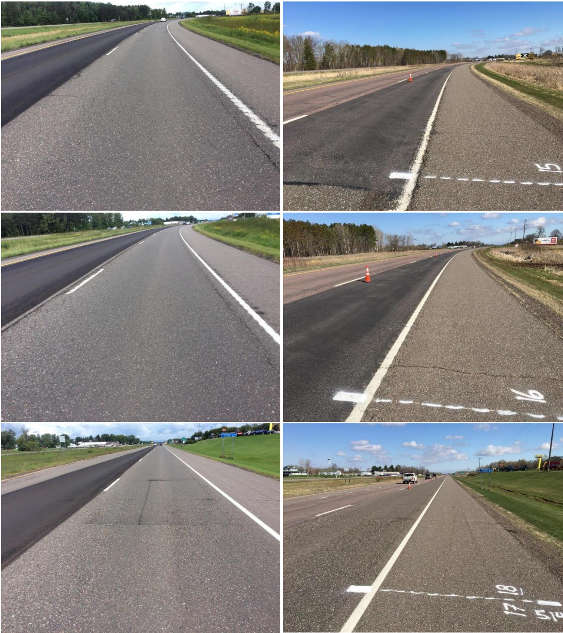
Controls: Cell 169015 (top), 169016 (middle), 169018 (bottom) inspected in 2016 (left) and 2020-21 (right).
