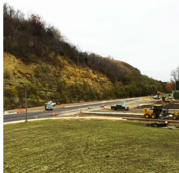
View from Oct. 31, 2017, where the button-hook ramp will meet a new traffic signal at Highway 61.
