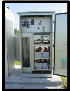
WITH BATTERY BACKUP
