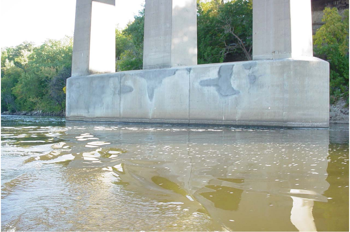
Photograph 3. View of East Pier, Looking Northeast. Note the Spall Repair.
