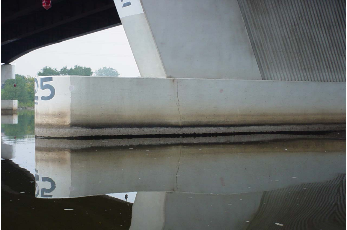
Photograph 5. View of Pier 3 Crack at Downstream Quarter Point, Looking West
