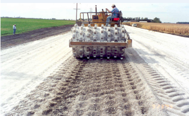
Fly ash was used as a stabilizing agent in the reconstruction of a road in Waseca County
