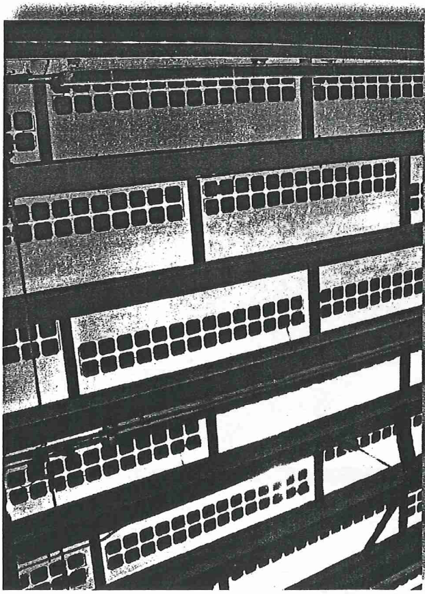
An integrated solar PV system installed in the skylights at the Marjorie McNelly Conservatory at Como Park in St. Paul
