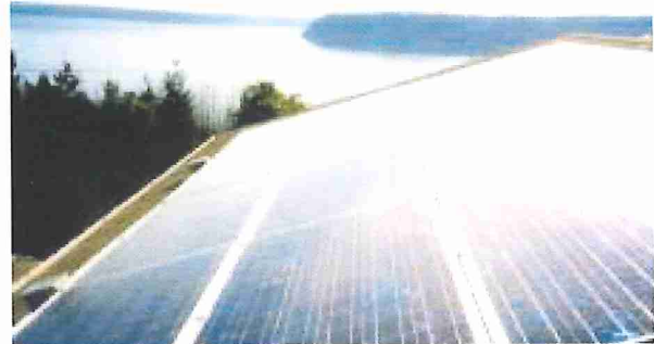
5 KILOWATT GRID-TIED PV SYSTEM
