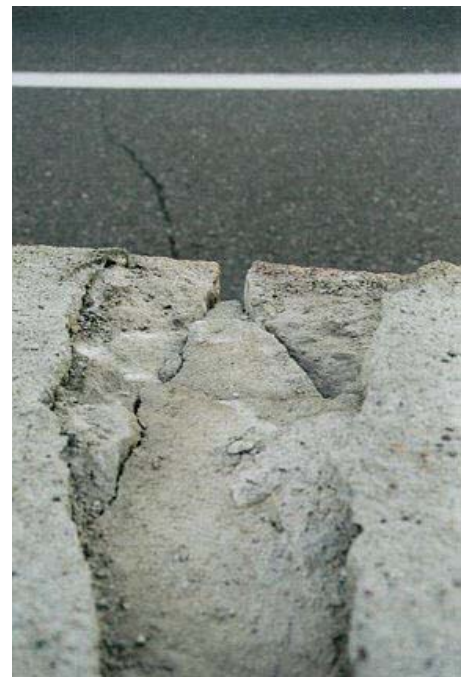
17. Close-up View of Missing Mortar and Condition of Underlying Stone Joint
