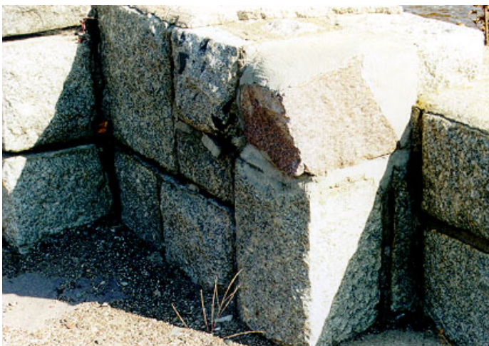
13. Patched End Caps ( spalled mortar topping above sloped stone patch and loose mortar behind )
