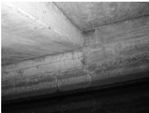
Figure 7. Cracks in the south abutment breastwall near the west construction joint. The upstream side of the wall is to the right in this photo. The lower original slab functions as a hydraulic constraint inside the bridge.
