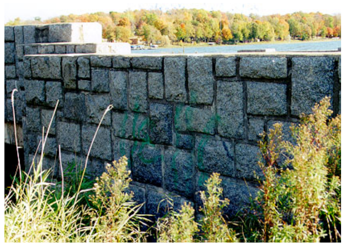
18. Graffiti on West Wall
