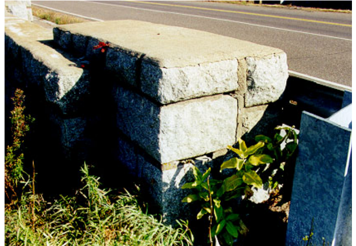
14. Wall End showing Poor Mortar Conditions and Overgrown Vegetation
