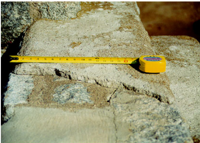
11. Mortar Topping at Walls ( broken and spalling )
