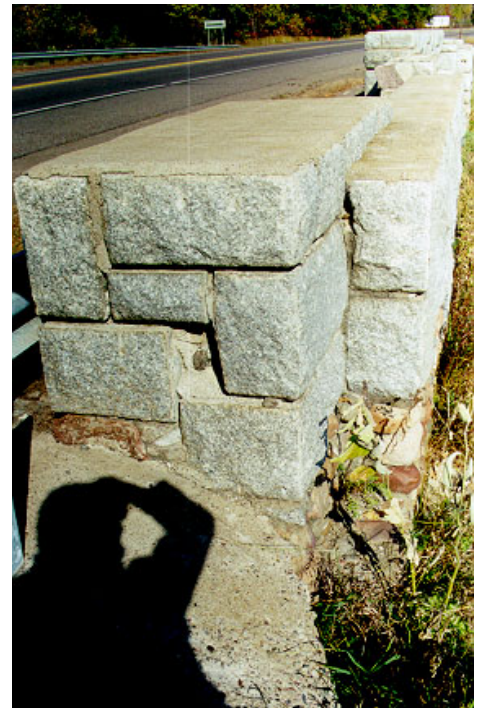
10. Missing Stone and Poor Mortar
