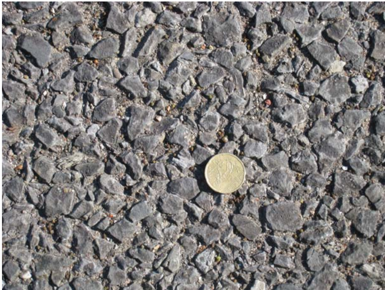
Figure 4.2. Close-up of the porous asphalt surface of the A12 motorway. Note fines infiltrating the porous asphalt surface on the edge of the traffic lane (SHRP2 2009).
