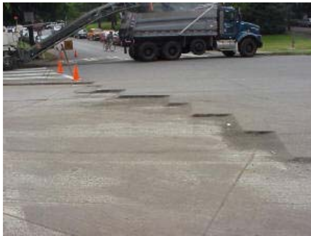
Figure 3.1. Milled road showing complete removal of the HMA overlay to expose the PCC slabs beneath (WSDOT).
