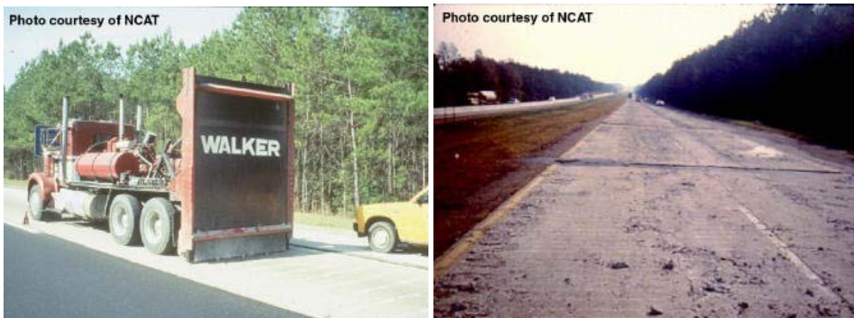
Figure 3.4. At left, guillotine hammer used for cracking and seating PCC; at right, PCC pavement after cracking and seating with guillotine hammer (WSDOT)
