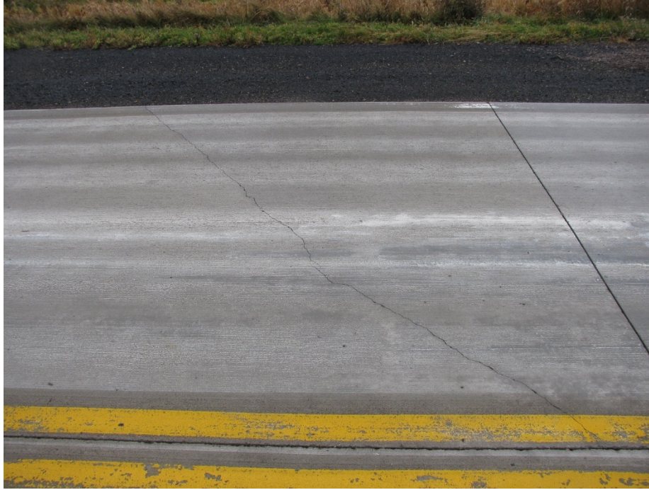
Figure 22- Cracking occurred on inside lane at Cell 138
