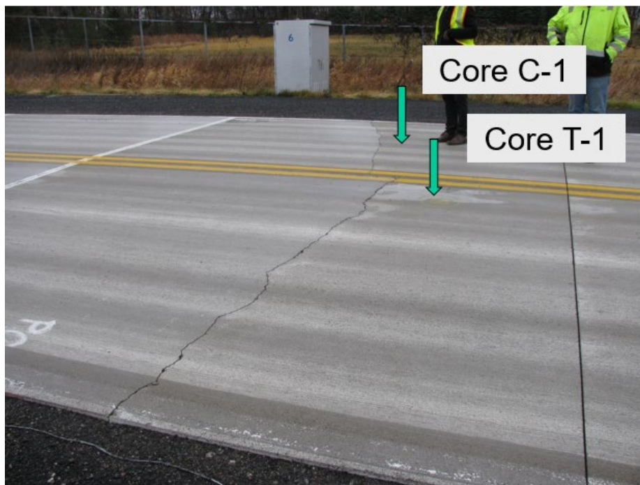
Figure 25- Distress in form of cracking near the wheel path at Cell 238
