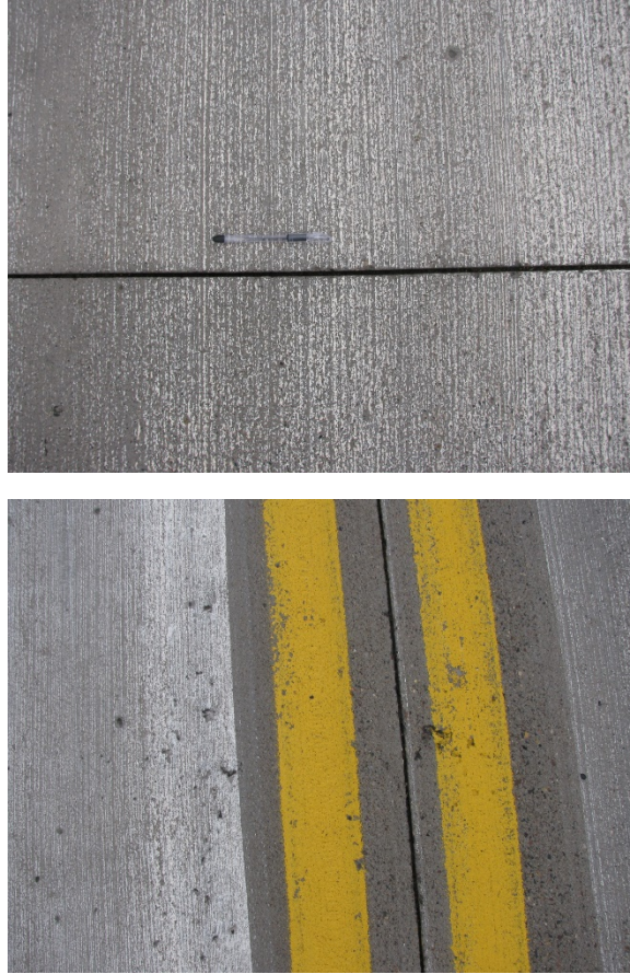
Figure 29- Typical surface quality at Cell 138 (top), and finishing issues observed at Cell 238 (Bot.)
