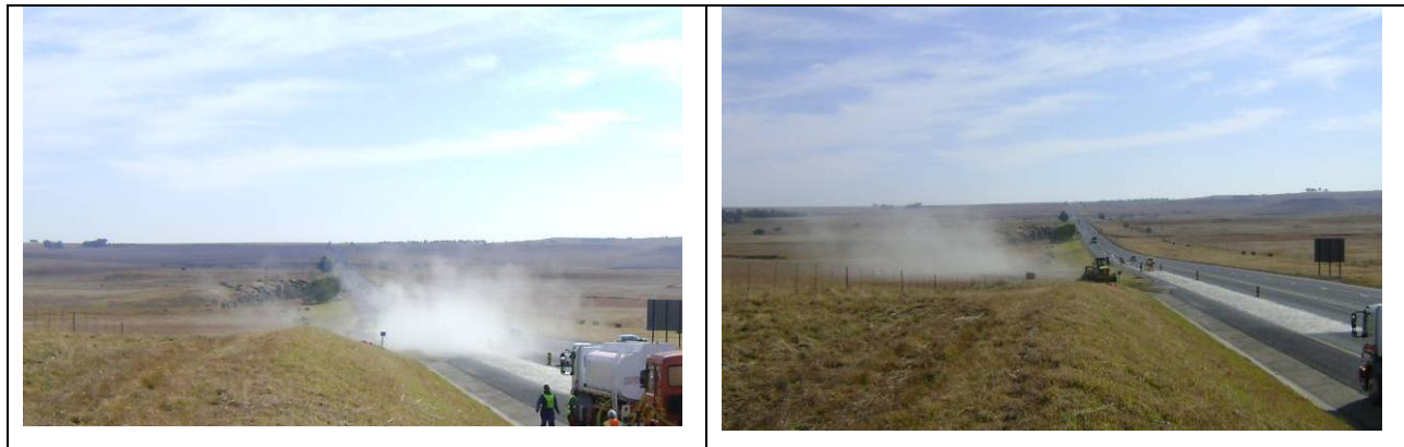
Figure 7.2: Cement loss by wind.
