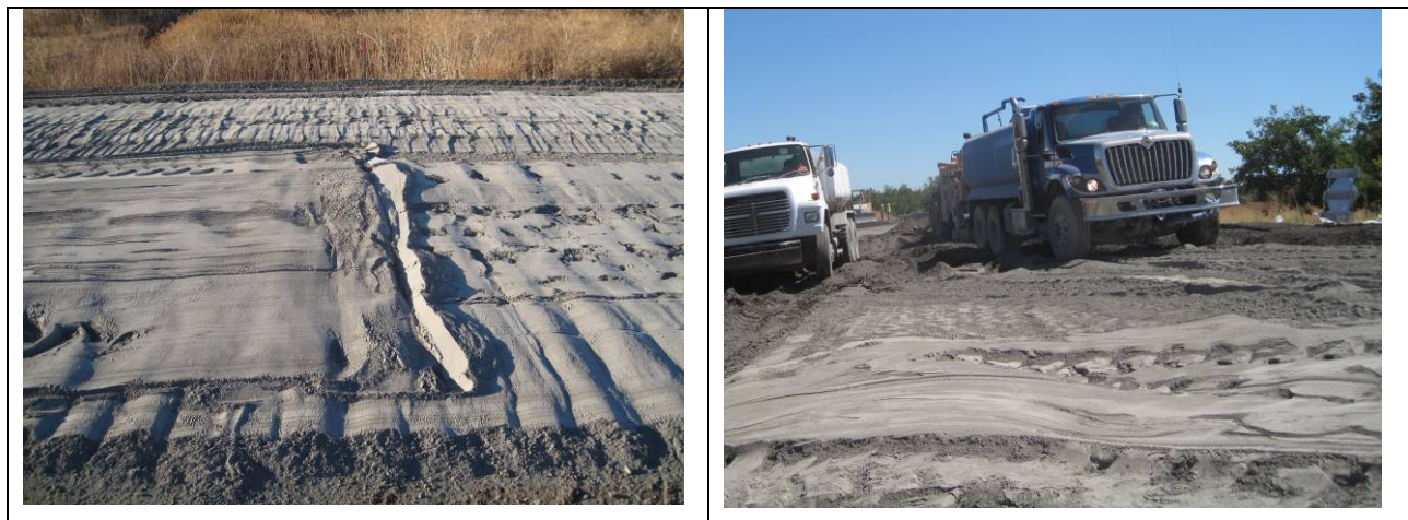
Figure 7.3: Uneven distribution of stabilizer on road surface.
