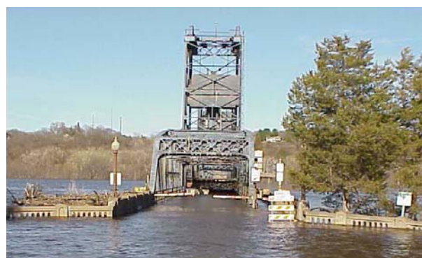
FIGURE 2-8 FLOODED LIFT BRIDGE (2001)
