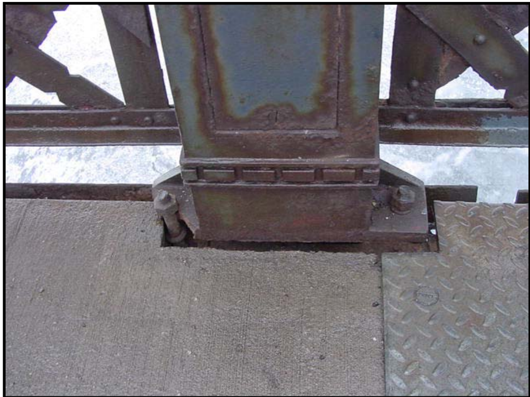
Photo 14: Broken Newel Post Anchorage Flange
