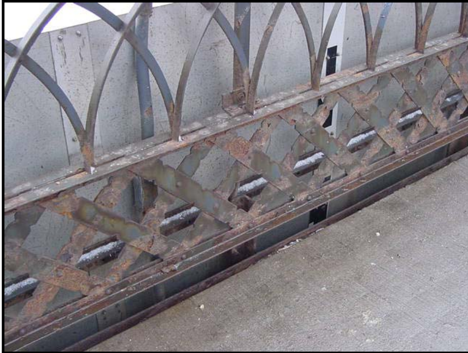
Photo 10: General Corrosion of Original Railing Cross-bar Pane
