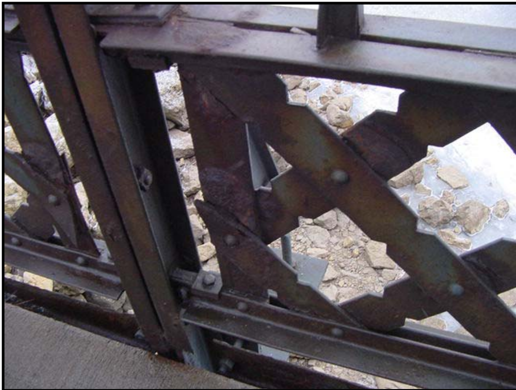
Photo 12: Corrosion of Original Railing Cross-Bars
