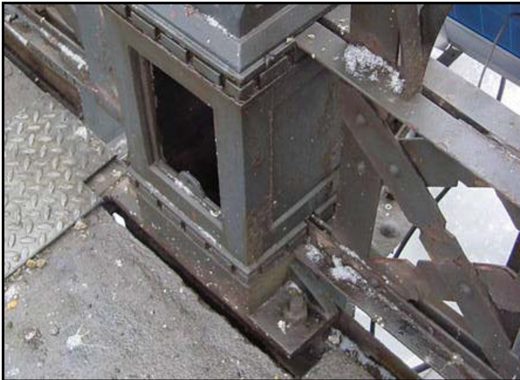
Photo 8: Newel Post Hand-hole – Missing Cover Plate
