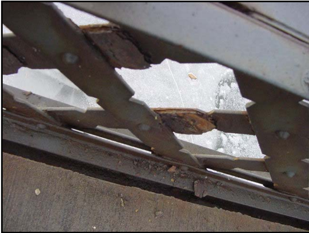
Photo 11: Corrosion of Original Railing Cross-Bars
