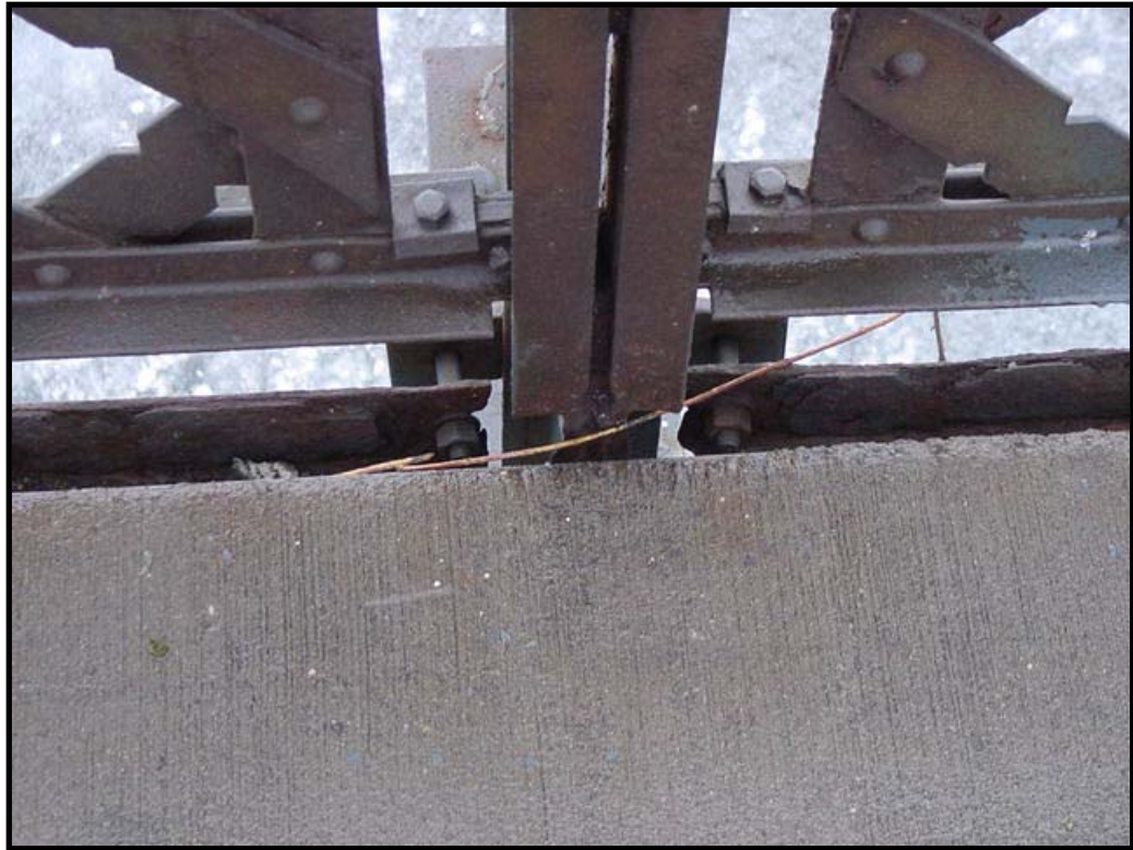
Photo 13: Substantial Section Loss to Rail Post Flanges Due to Corrosion
