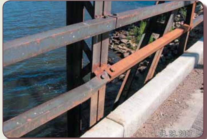
North Railing—Bent and Corroded Members
