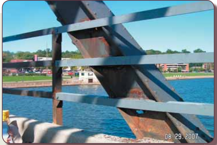
Truss, Portal Member—Steel Section Loss
