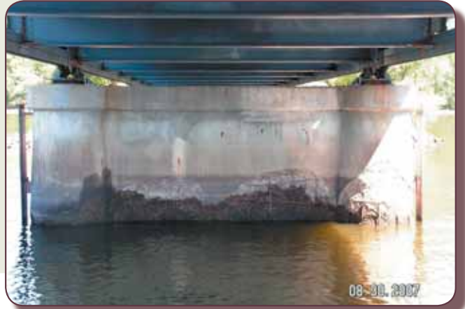
Pier 8—Concrete Deterioration
