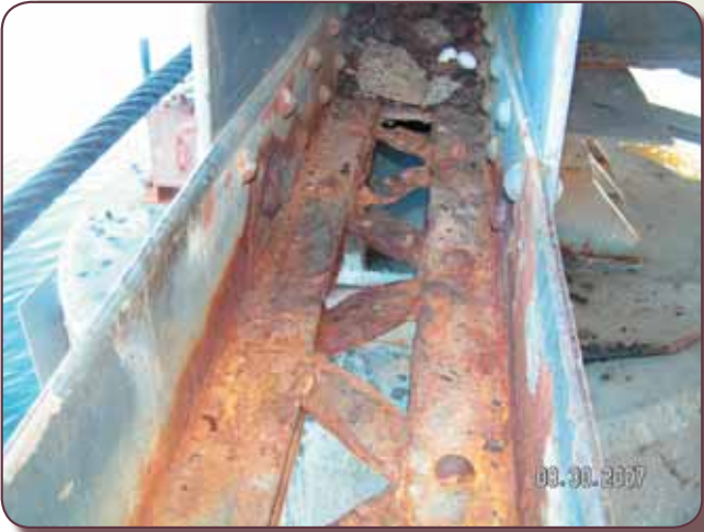
Corroded Areas of Lower Truss Chord
