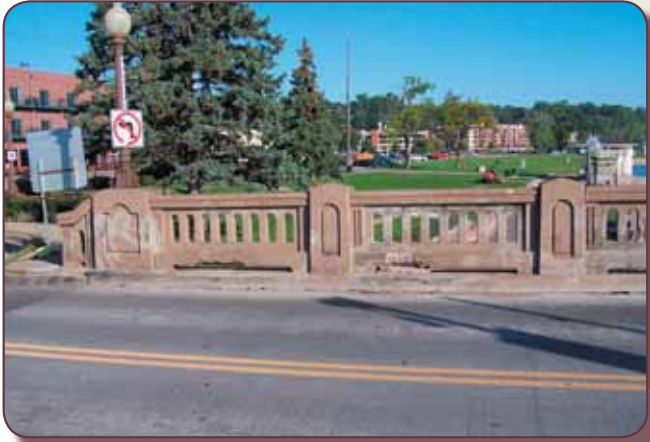
Span 1 Ballustrade—Concrete Spalling
