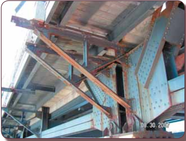
Corroded Sidewalk Support Bracket
