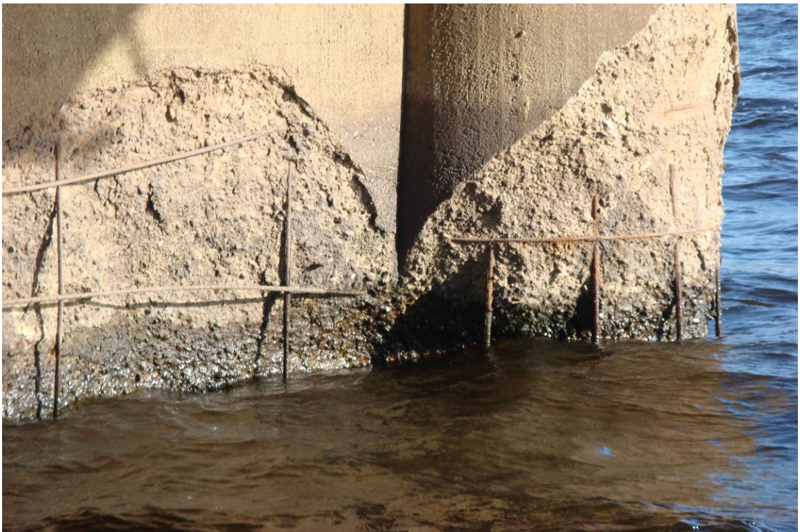
Photograph 8. View of the Concrete Section Loss on the West Face of Pier 8, Looking Southeast.
