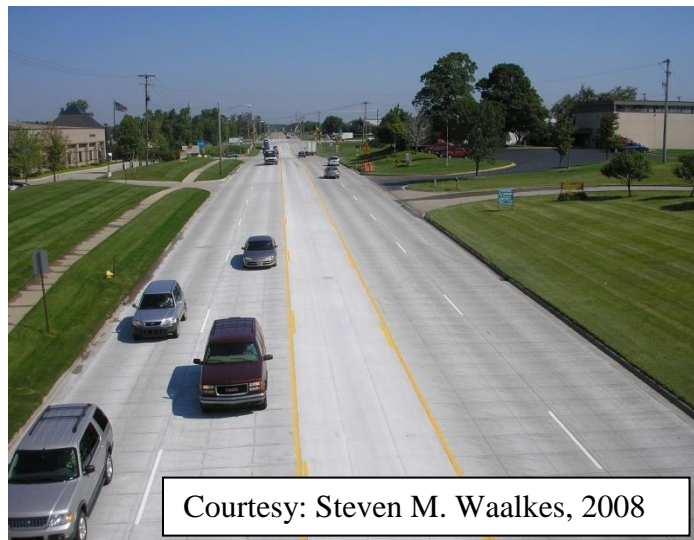
Figure 48: Condition of the UTW after two years (2008).
