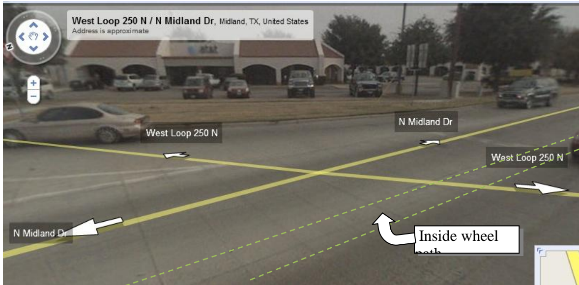
Figure 40: UTW at the intersection of LP-250 and Midland Drive at Odessa District. (Google Street view (February/2009))
