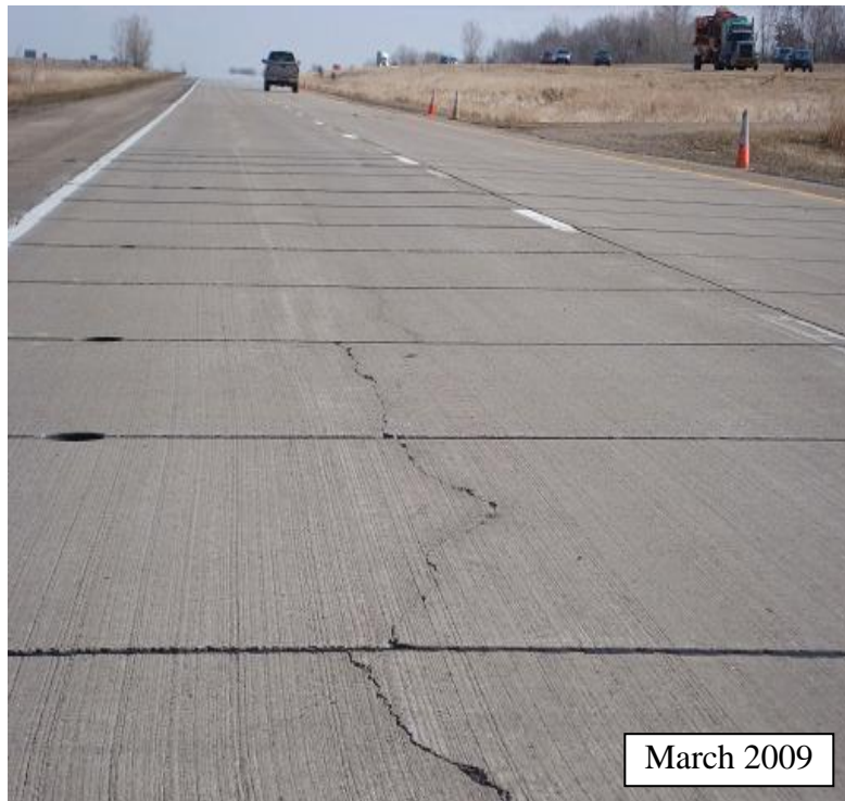
Figure 20: Longitudinal cracks in Cell 97.
