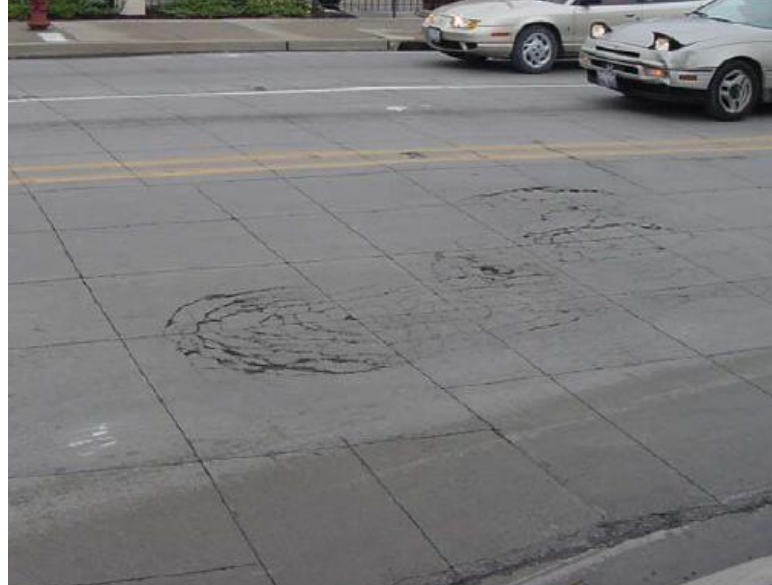
Figure 44: Distressed panels at the intersection. (Winkelman, 2005)
