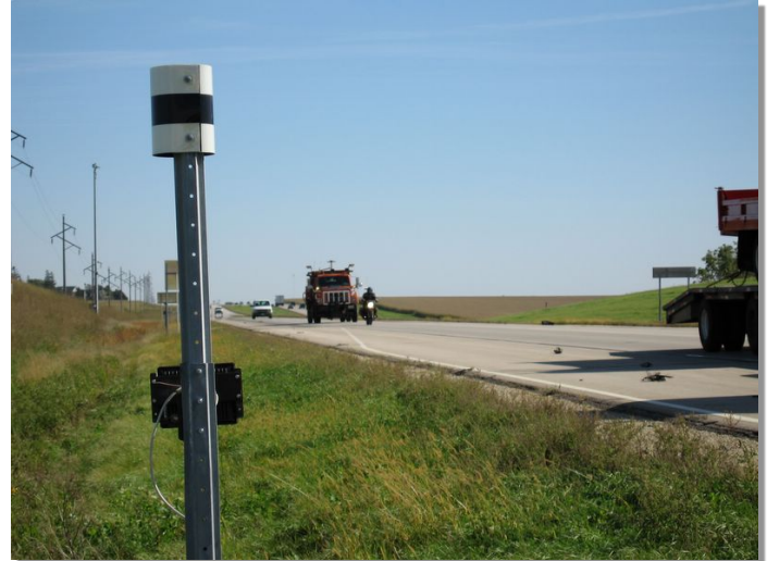
The CICAS detector as installed at Highway 52.
