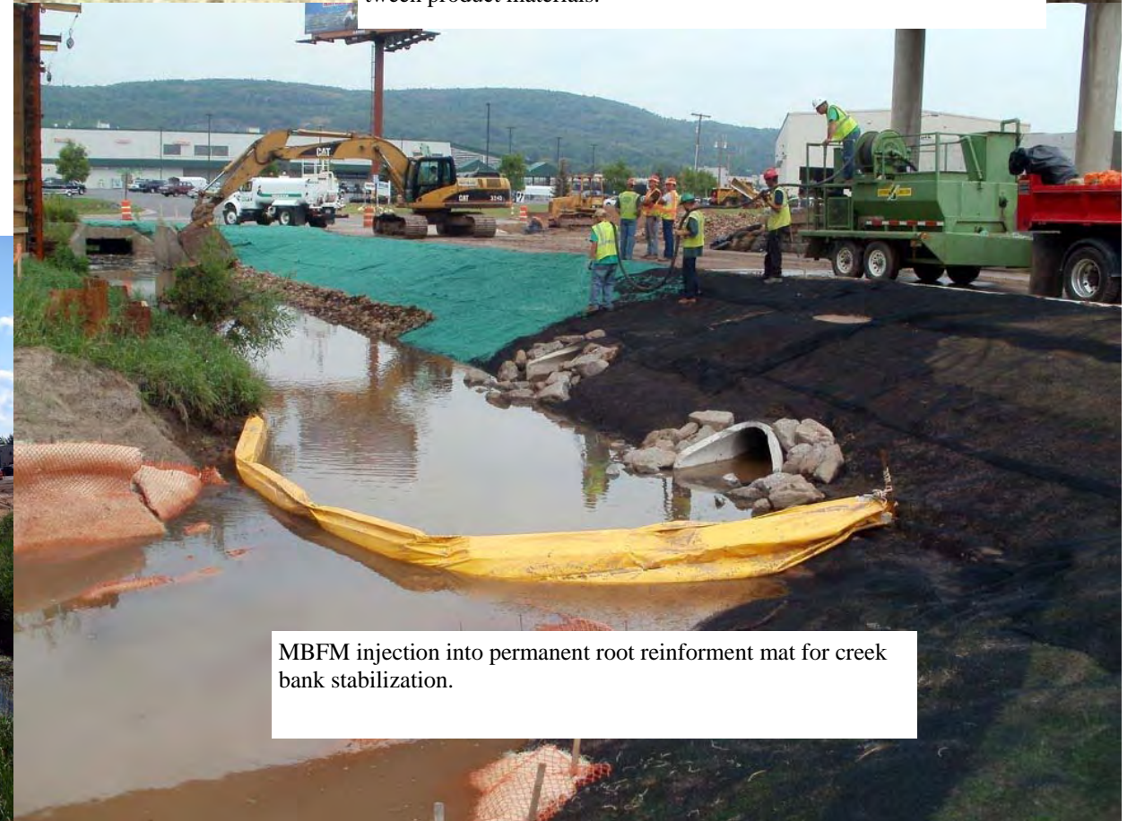
BFM first lift placement on properly prepared seed bed. Blanket installed at top of slope in rural section to prevent rill formation. Ditch section is low gradient between driveway access. Otherwise, appropriate blanket should be installed to wetted perimeter. BFM does a fantastic job anchoring blanket and provides a smooth transition between product materials.
