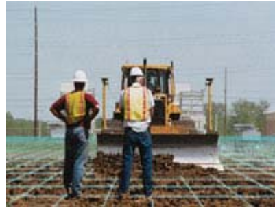
Precision. Operators like GPS dozer control to guide them for rough grading and go fully automatic for fine grading. (Photo courtesy of McAninch Corp)
