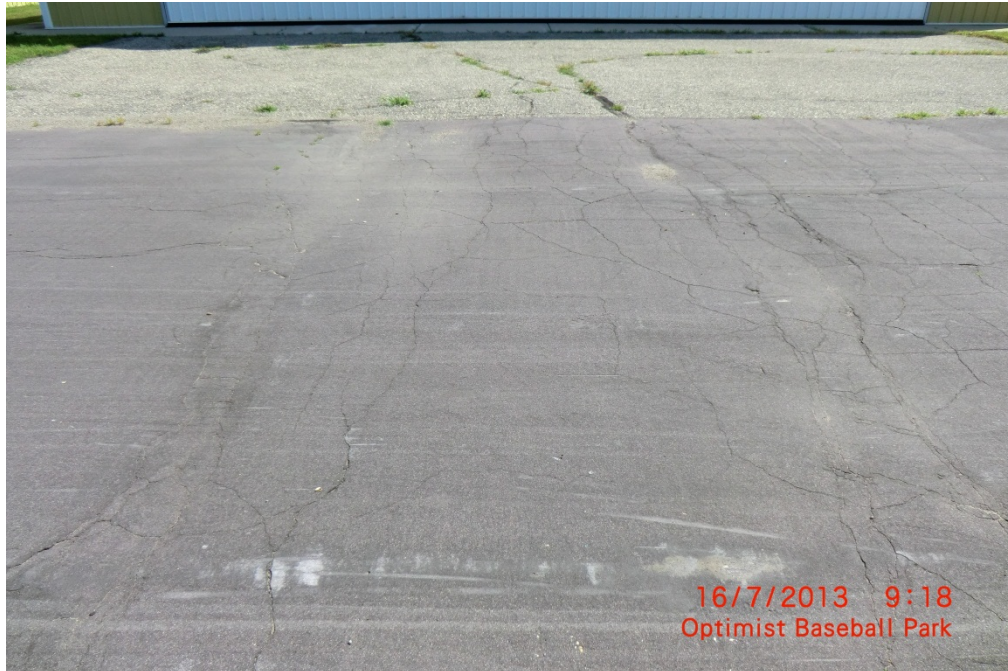
LJF TLA 001 (Medium-Severity Alligator Cracking & Low-Severity Rutting)
