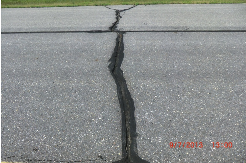
AXN PTB 001 48L (Low-Severity L&T Crack)
