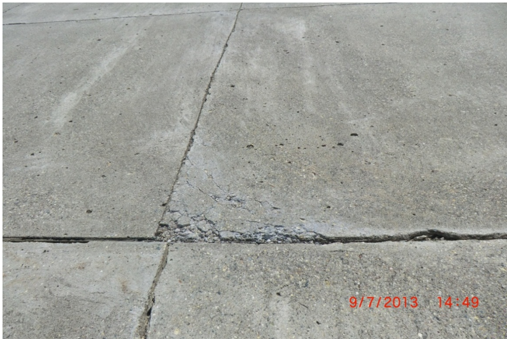
AXN APA 002 (Medium-Severity D Cracking)
