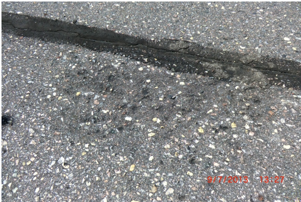
AXN PTB 001 52H (High-Severity Raveling)
