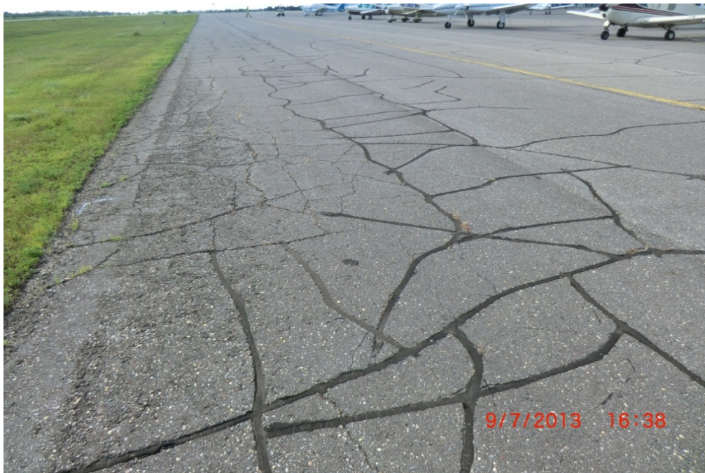
AXN APA 001 (High-Severity Block Cracking and Raveling)
