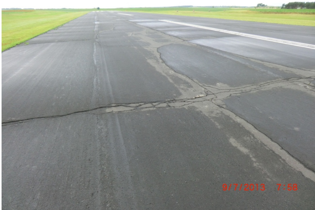
14Y RY1634 001 (PCI = 58, prior to rehabilitation)
