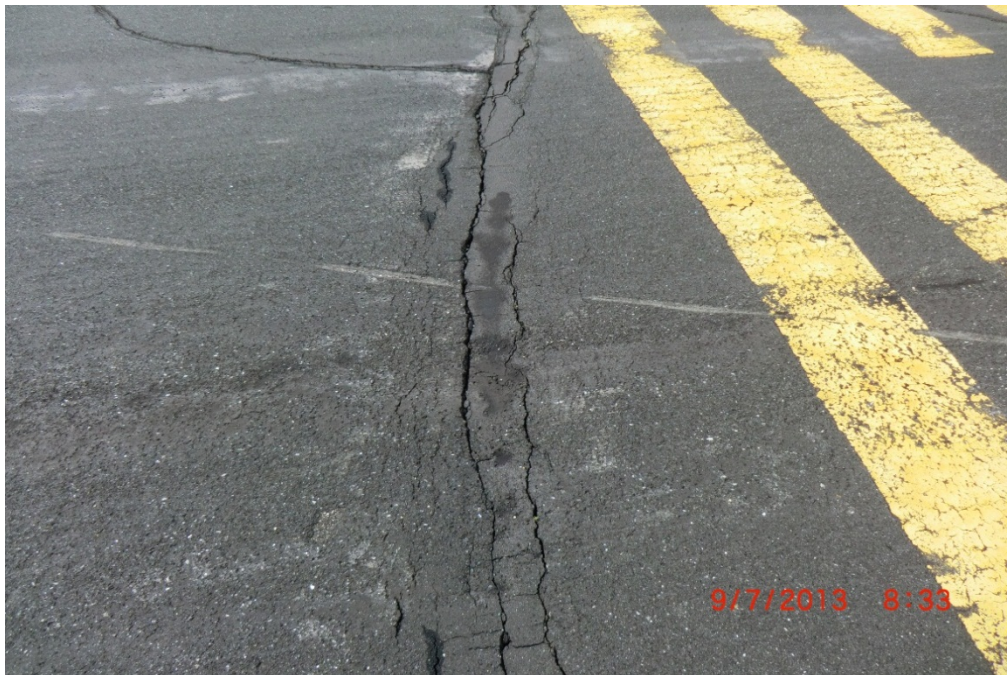
14Y CTA 001 (High-Severity L&T Crack, prior to rehabilitation)
