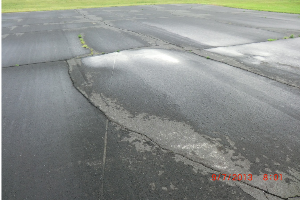
14Y RTA 001 (PCI = 53, prior to rehabilitation)
