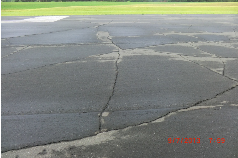
14Y RY1634 001 (PCI = 58, prior to rehabilitation)
