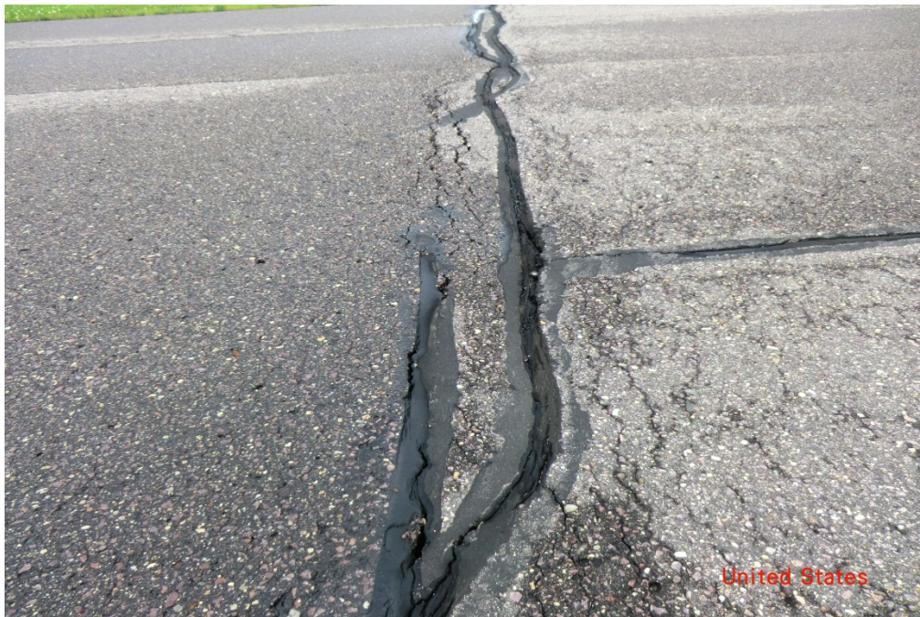
1D6 RY1230 001 Alligator Cracking (PCI = 60)
