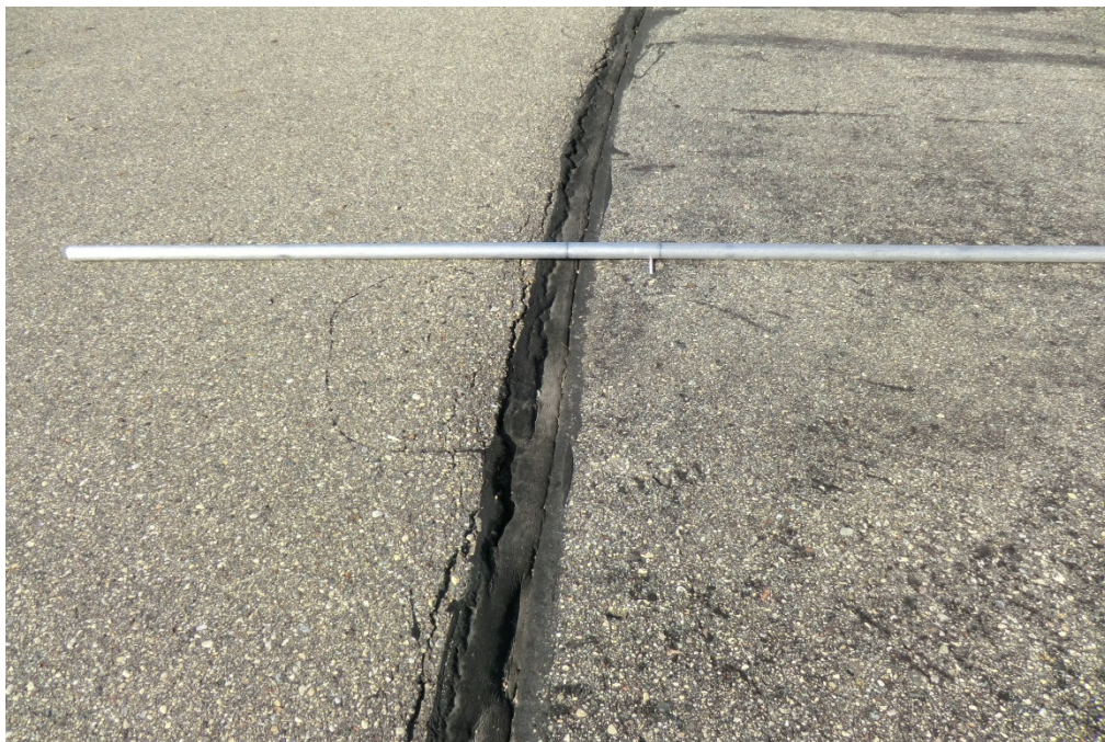
SBU TLB L & T Cracking
