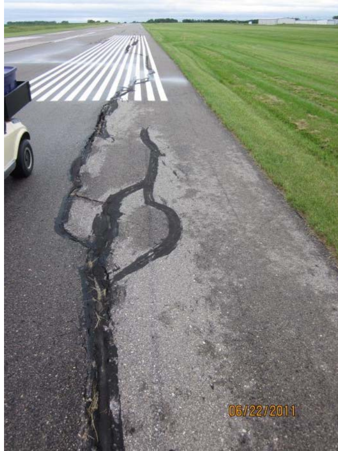
Y63 RY1432 major crack near edge of runway.
